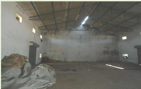
Leaking roof of godown, MLS Point, Jainath (Adilabad district)
