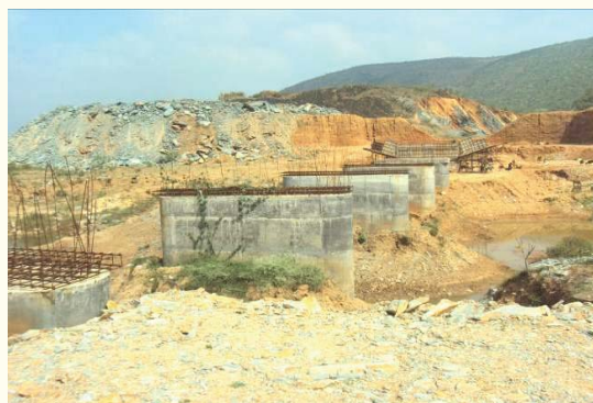
Non completion of CM & CD 21 works (Aqueduct)
